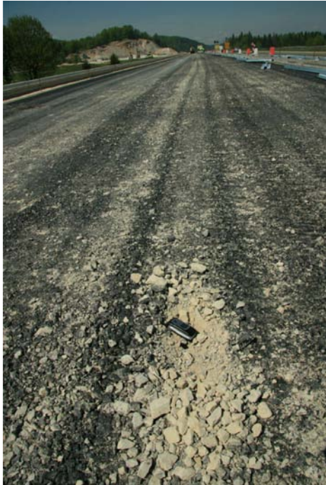
Figure 2 Damaged course on the segregated surface
