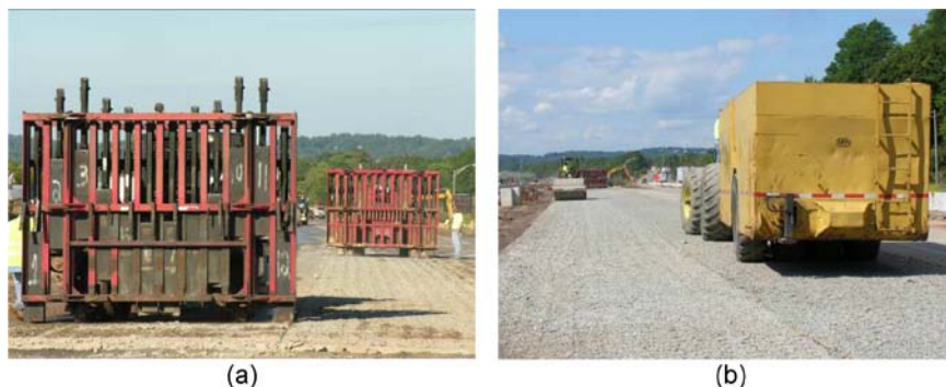
Figure 1 MHB rubblizing PCCP (a) and compaction of rubblized PCCP by z-pattern and pneumatic tire rollers (b).
