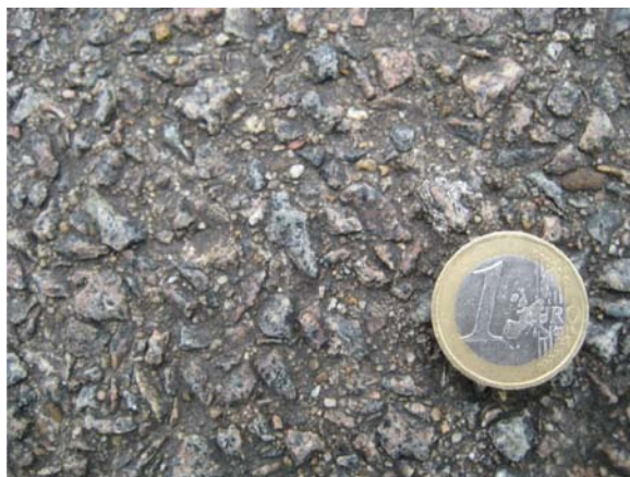
Figure 2 Surface of the concrete pavement
