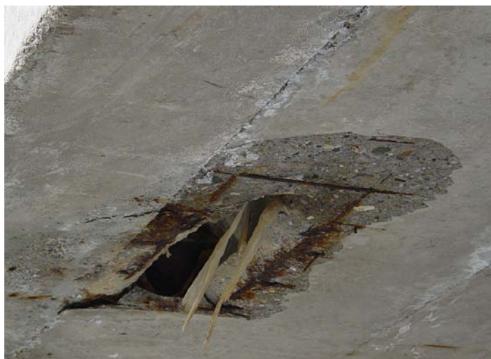
Figure 3 Pavement structure damage
