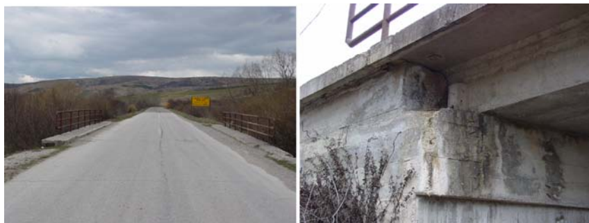
Figure 4 View of the bridge and water penetration through pavement structure
