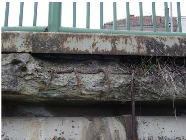
Figure 6 Reinforcement corrosion on pathway cantilever
