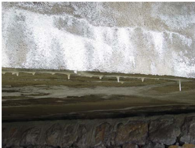
Figure 7 Calcification due to water penetration through the structure
