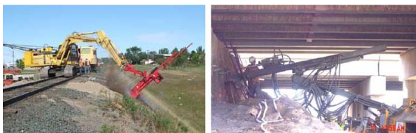
Figure 3 Installation of soil nails from the top of existing railway embankment using Soil Nail Launcher technology [12] (left) and installation using mobile rig under a bridge end-span (right).
