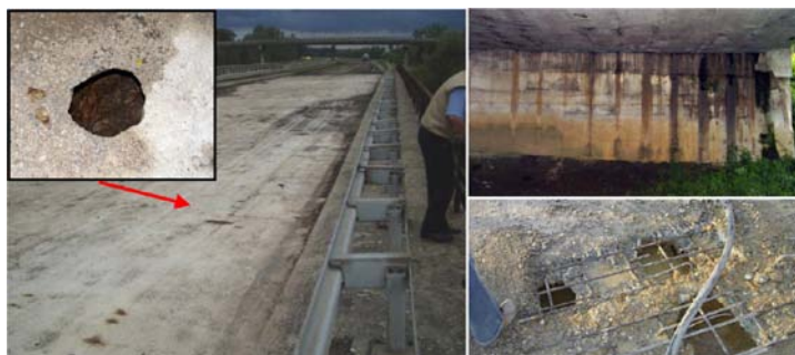
Figure 8 Visible wholes after removing asphalt surfacing and waterproofing, leaking on abutments through all 12 deck slab voids, after removal of levelling course concrete is sipping into voids[4]
