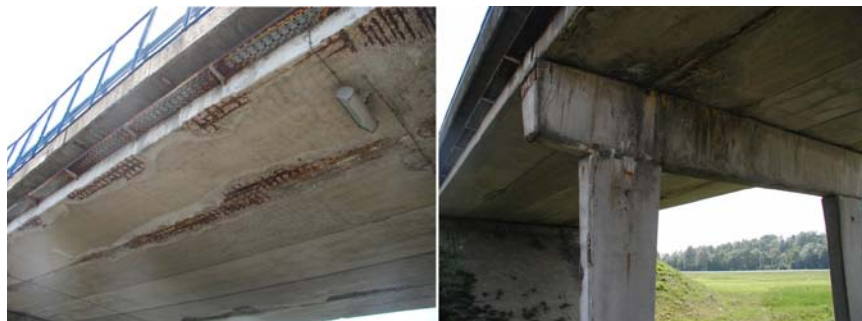
Figure 2 Overpass junction 'Ivanič Grad' on highway Zagreb-Lipovac: severe reinforcement corrosion and leaking [2]
