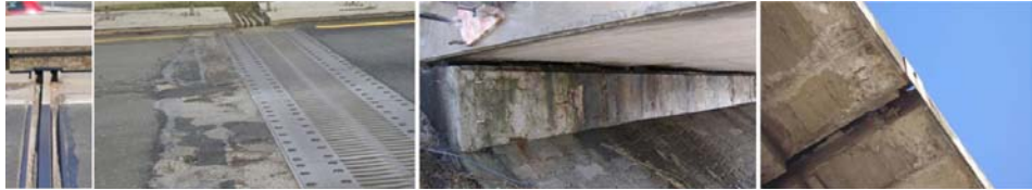
Figure 10 REJ without sealing filled with debris, denivelation of asphalt, severe leaking on abutments and cantilever soffit underneath REJ
