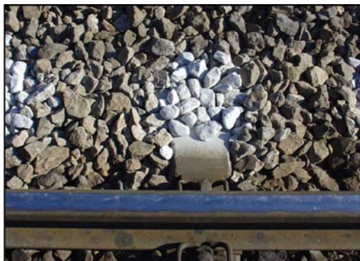
Figure 13 “Median” level of ballast degradation
