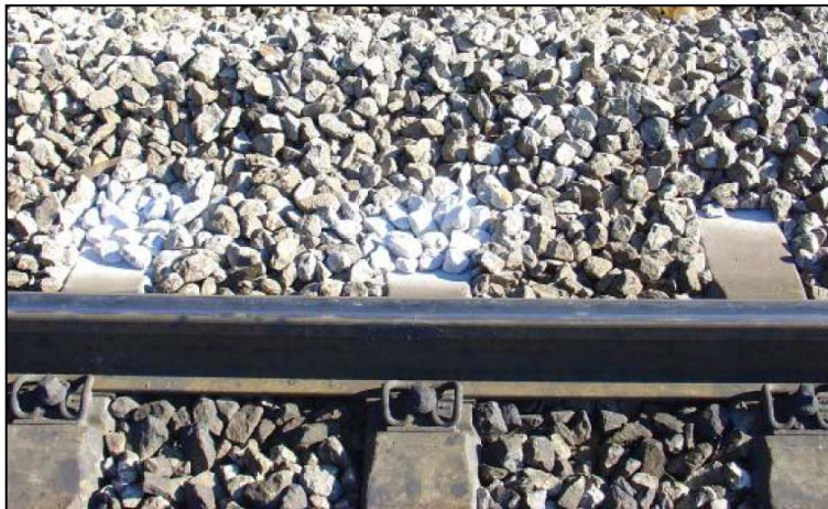
Figure 2 Settlement of the concrete sleepers
