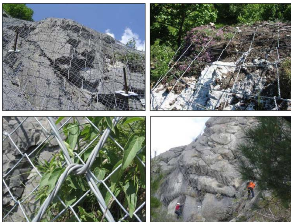
Figure 3 Rock protection with high-tensile spiral rope nets combined with rock bolting (on the right under corner protection of a rock mass in Brzjet, Croatia).
