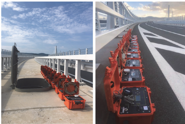
Figure 14 Synchronised current interrupters used to simultaneously interrupt all 20 CP units
