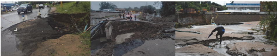
Figure 7 Structural collapse and overtopping along Stapleton road [13-15]
