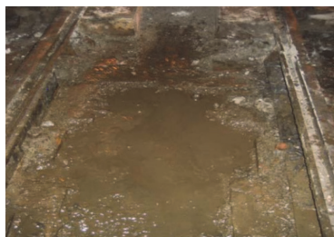
Figure 4 Condition in closed track structure during the most period in a year
