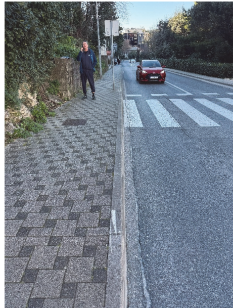
Figure 4 Pedestrian crossing no. 2 – bad practice example – no dropped kerbs
