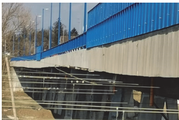
Figure 4 Differential settlement of the AB span of the northern viaduct resulting from pier settlement (S2–S6) due to seismic ground movement [2]
