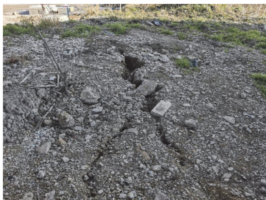
Figure 2 Seismic-induced soil crack between piers S5 and S6 [2]
