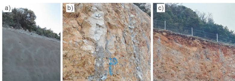
Figure 3 Protection on slope: a) type 2, b) modified type 3, c) rockfall protection barrier
