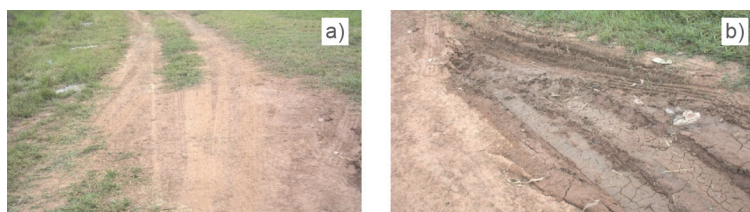
Figure 7 a) Unpaved access road to UNICAMP, b) deep depression on the side of the same road
