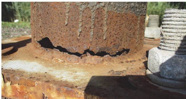
Figure 5 Corrosion degradation on poles base [18]
