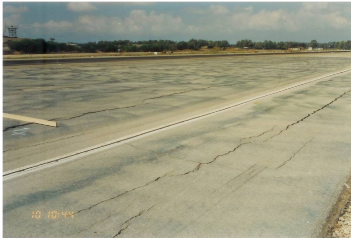
Figure 1 Severe longitudinal cracking and differential settlement and heaving taking place on the surface of a pavement based on an expansive clayey subgrade
