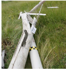
b) The column after the impact – vehicle speed was reduced to 60 km/h
