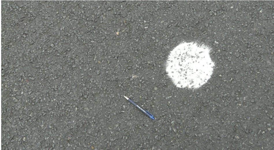
Figure 5 Surface aspect of micro-surfacing after one year of service
