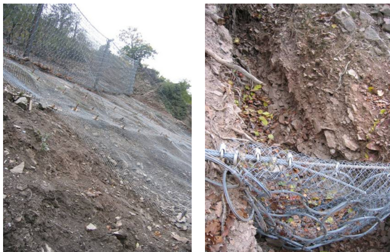
Figure 6 Slope stabilisation for the loose deposited material (left) and small debris brake at a gully to reduce the flow energy level (right).
