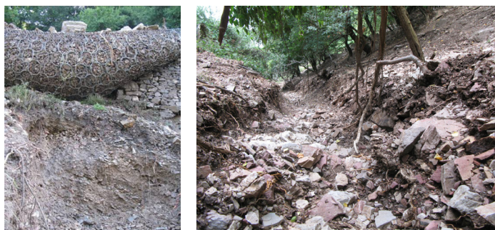
Figure 2 Installed ring net barrier of 2005 filled after the event in July 2008 (left) and gully after the same event (right).
