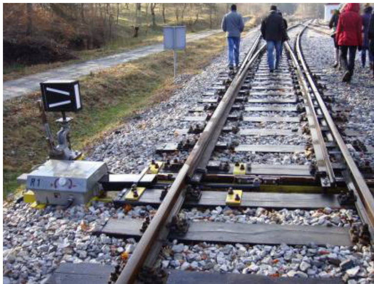
Figure 3 Disconnector switch on special track
