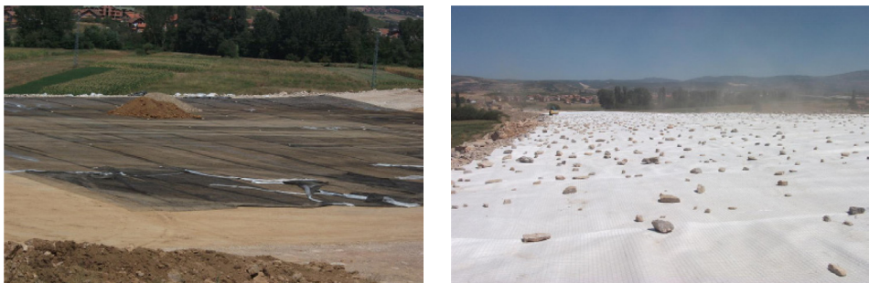
Figure 9 The geogrids were placed over the full embankment width, starting at app. 373 m altitude, which is approx. 0.5 m above the 100–year flood level. A combigrig was installed underneath the road base course over a width of approx 30.9 m. A combigrig was installed transversely to the road axis, with an overlapping of a min 300 mm in both adjacent and longitudinal directions.
