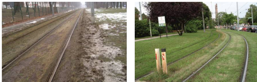
Figure 6 Damages by winter service: Grass sods peeled from the track and dumped alongside the track (left). View of the test field at Lainz before re-cultivation (right)
