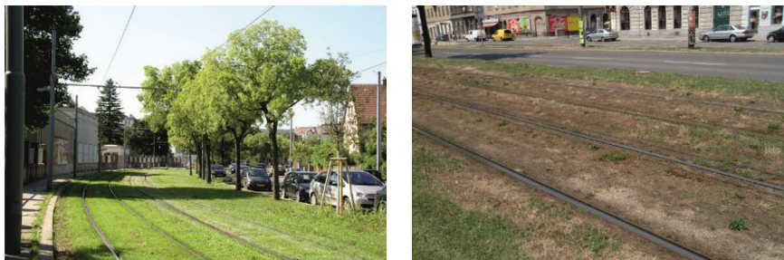
Figure 2 Existing green track in good (left) and unsatisfactory shape (right)
