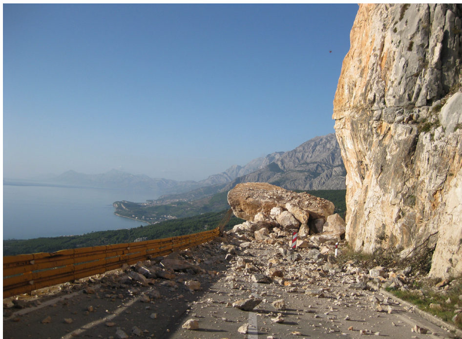
Figure 1 The rockfall on the D512 state road
