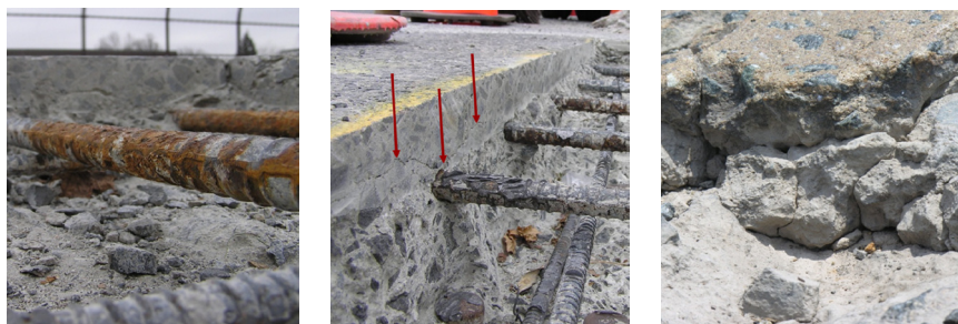
Figure 1 Rebar corrosion, delamination and concrete degradation.
