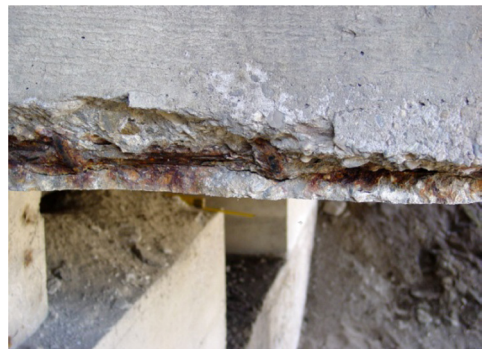
Figure 3 Exposed, corroded reinforcement
