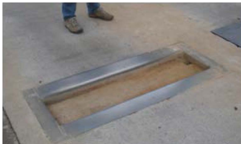
Figure 5 Detail of the pothole track
