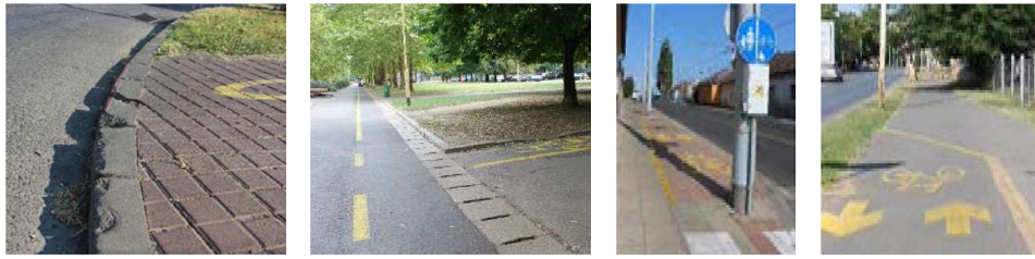
Figure 5 Bicycle paths design and construction irregularities in the city of Osijek
