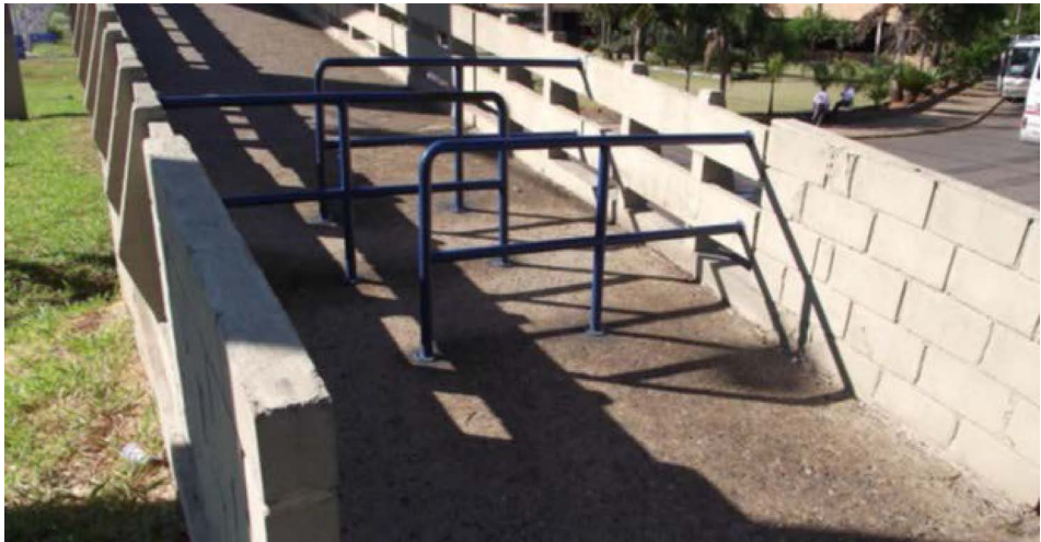
Figure 5 Obstruction in a walkway giving access to a stopping point located on Zeferino Vaz highway, shown in Figure 6
