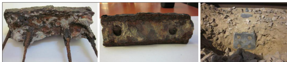
Figure 2 Severe corrosion on anchor plate & rebar, on anchor plate
