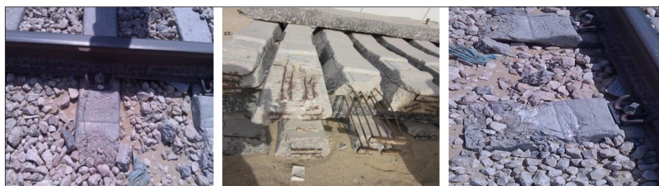
Figure 1 Cracked and Corroded Concrete Sleepers (km 19, 25, 31 & 37)
