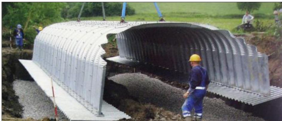
Figure 4 Erection of the corrugated steel structure with an attached support in the form of a flat sheet
