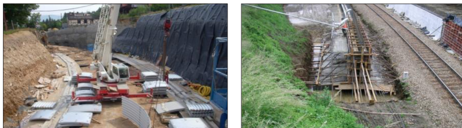
Figure 9 Soil-steel tunnel foundation on a beam grid / Solid foundation of a soil-steel structure
