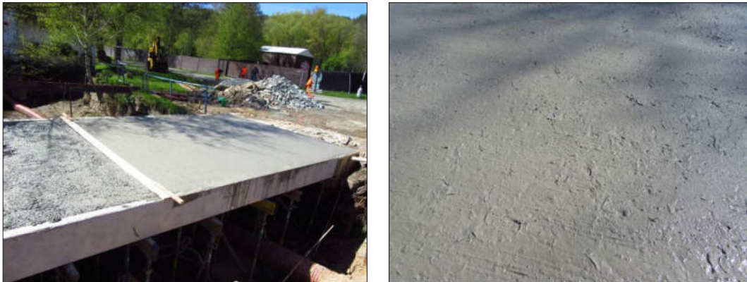
Figure 3 Left: Levelling of concrete surface. Right: Surface of fresh concrete after burlap dragging.
