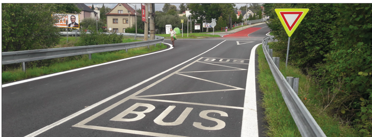
Figure 4 This part of the road was reconstructed, including the new traffic signs. In this locality approximately 20 connections stop every day. But the design of the bus stop area including the access for the pedestrian was not done. According to the information there is not a plan to do it in the future – high risk.
