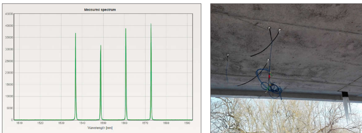
Figure 7 Pictures from the checking of the sensors. Left – measured spectrum of four FBGs in GFRP sensor. Right – damaged connectors of SAF sensors
