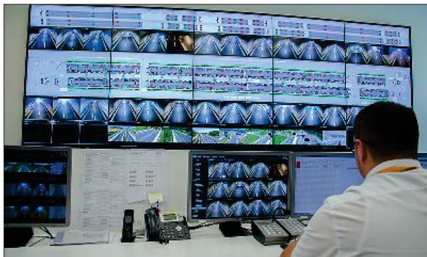
Figure 4 Center for Maintenance and Control of Road Traffic FBIH- JP Autoceste [14 ]
