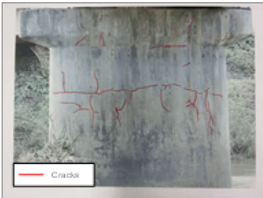
Figure 2 Diagnostic results of cracks by staff inexperienced in bridge inspection
