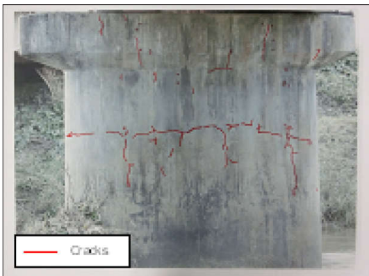
Figure 3 Diagnostic results of cracks by staff inexperienced in bridge inspection
