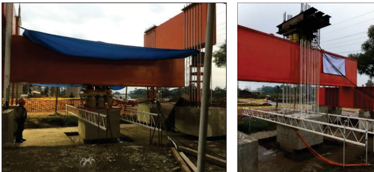
Figure 1 Structural arrays of girders and jacks for the compression and tension load tests
