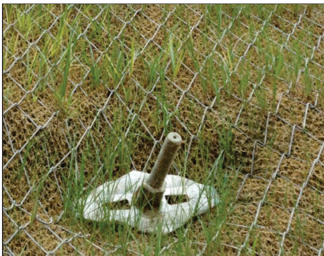
Figure 10 TECMAT erosion control mat in combination with a TECCO® G65/3 high-tensile steel wire steel wire mesh in the area of soil nailing
