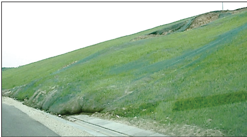
Figure 2 Slumping on an embankment with a slope at approx. 25°, secured with a geotextile/erosion control mat for greening without nailing
