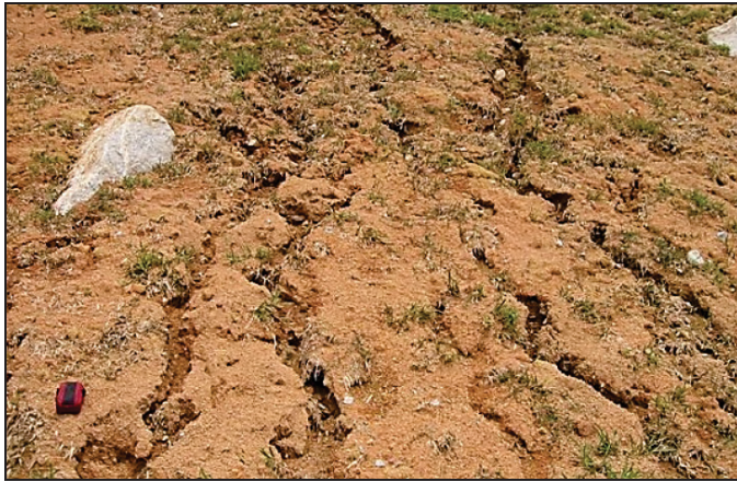
Figure 3 Erosion channels caused by the flow effect of the draining water, which remove the soil and reduce and/or prevent the growth of plants
