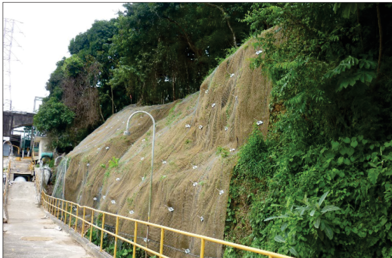
Figure 11 Secured rock embankment in Miraflores, Panama. Erosion protection mat and mesh could be adapted well to the irregular slope
