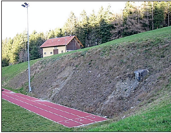
Figure 1 Ad hoc slumping on a slope in the grounds of a sports facility
