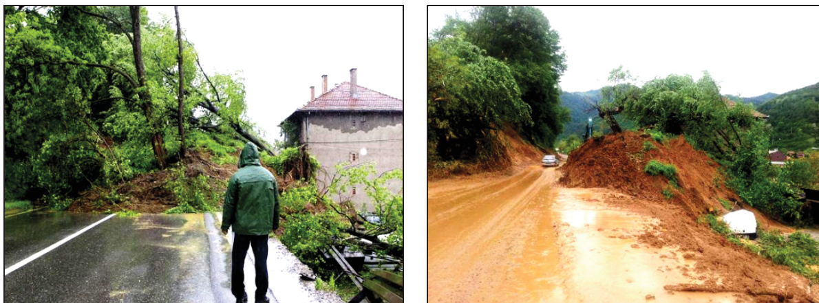
Figure 5 Landslide, Locations: Nemila, Main road M17, Topcic polje -Lasva km 3+880 (after floods in May 2014.)
