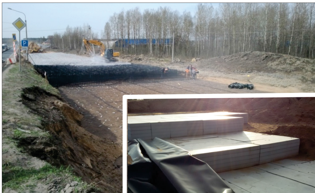
Figure 3 The initial stage of the geomattresses, geodrains installation – prototype (a) and geofoam blocks (b)
