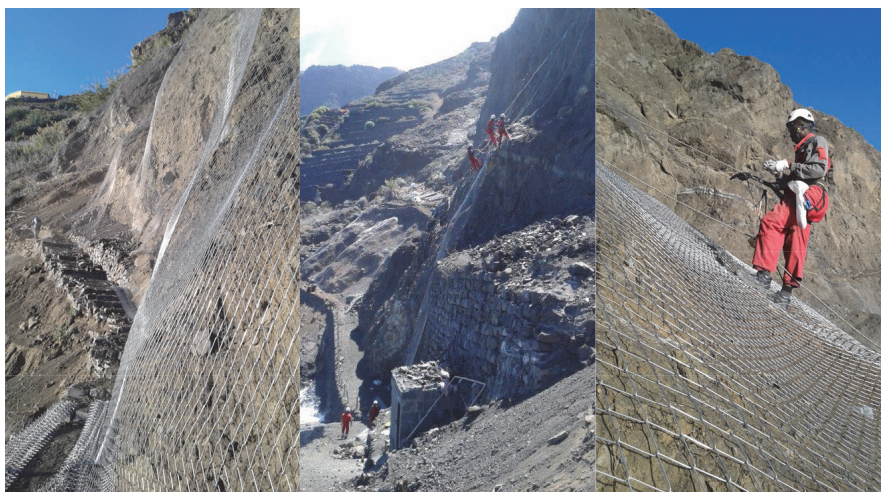
Figure 6 Installation of stainless steel on a rocky outcrop on La Gomera in 2015
