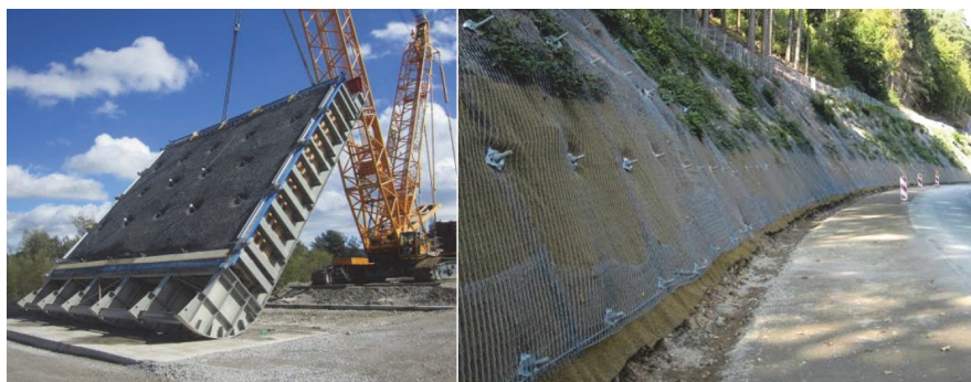
Figure 1 1:1 large field test to verify the RUVOLUM concept (left) and installed slope stabilisation project (right)
