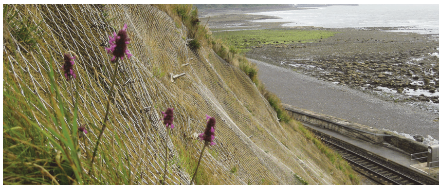
Figure 4 Stabilised soil slope above the rails, with high-tensile stainless-steel mesh. The proximity to the sea is evident as well as the exposure to constant salt spray.
