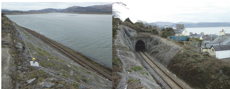
Figure 5 The exposure of the rail and the slope at Aberdovey tunnel approach (left) and stainless-steel mesh installation at tunnel portal (right).
