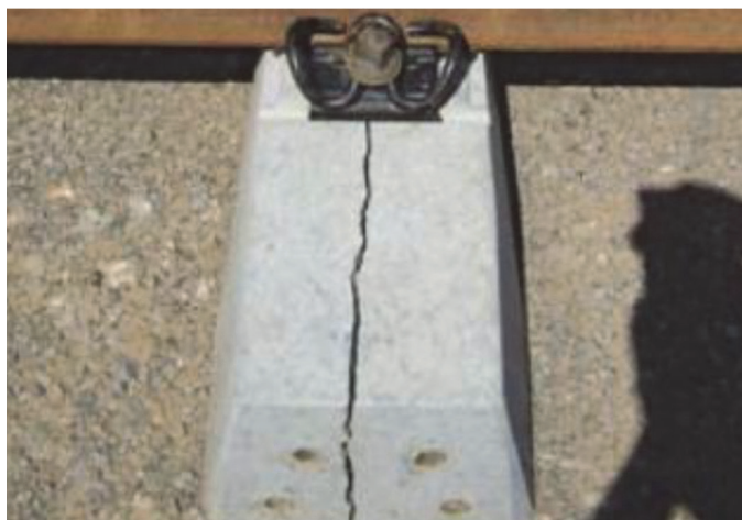
Figure 6 Longitudinal cracking on the concrete sleeper [5]
