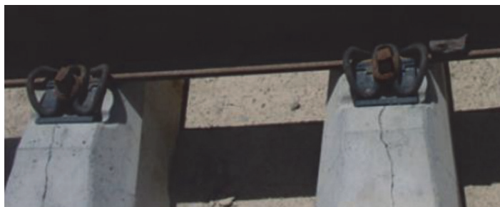
Figure 7 Longitudinal cracking in the concrete sleeper
