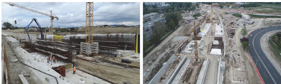
Figure 3 A phase of derived diaphragms and underpass (left) and derived diaphragms, underpass, and temporary road for traffic regulation (right)
