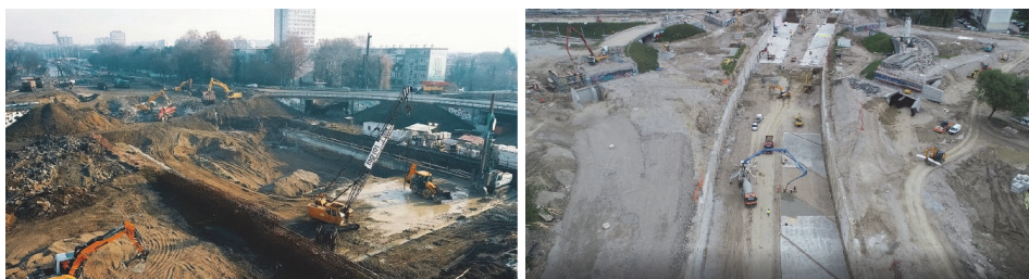
Figure 1 The diaphragm works for the protection of the construction pit (left) and peripheral drainage ribs (right)
