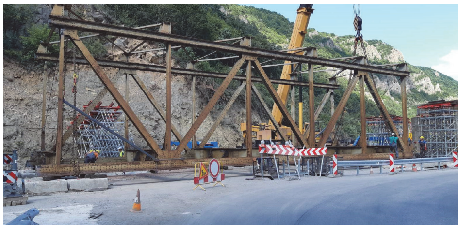
Figure 7 The middle part of the steel superstructure of the old bridge is lowered with two cranes
