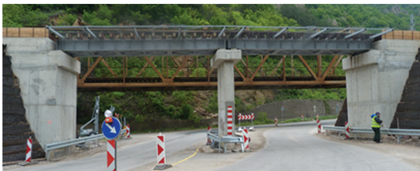
Figure 4 New temporary RW bridge – general view with the old riveted bridge in the background
