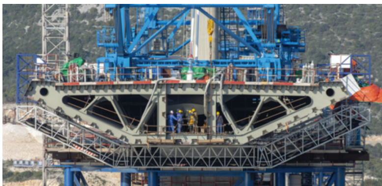
Figure 2 Standard cross-section of steel box girder with anchor box (March 2021) Source : CRBC
