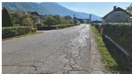
Figure 3 An example of deficient and poorly maintained transport infrastructure
