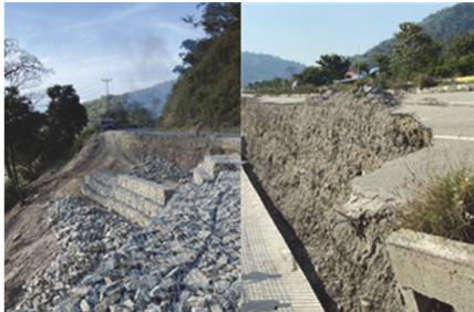
Figure 1 Slope failure along the main road
